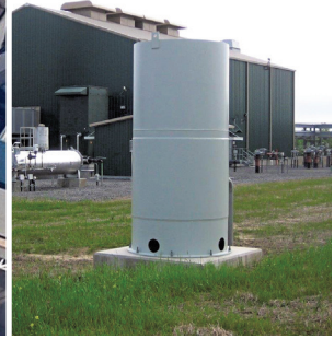
» Vent blowdown silencer at a gas compression station
